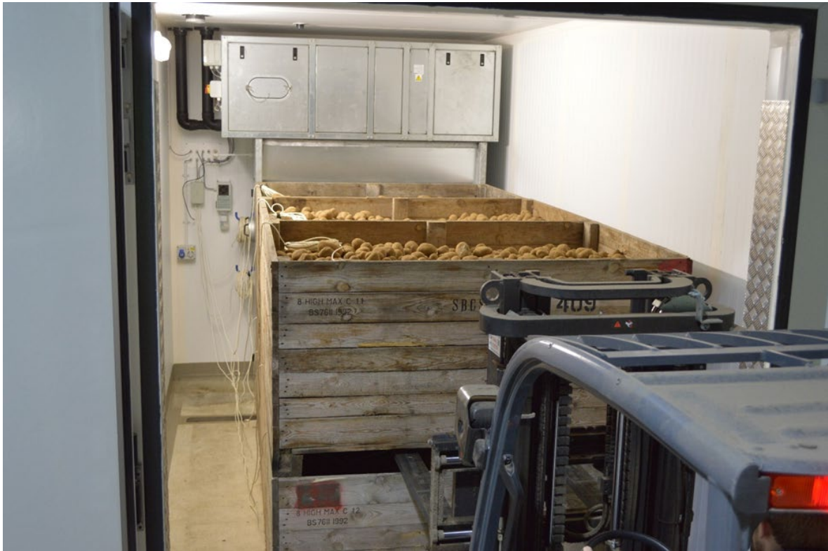
Fig. 1. Boxes stacked two high, three deep against a plenum, at the back of the store, for positive 'letterbox' ventilation.
