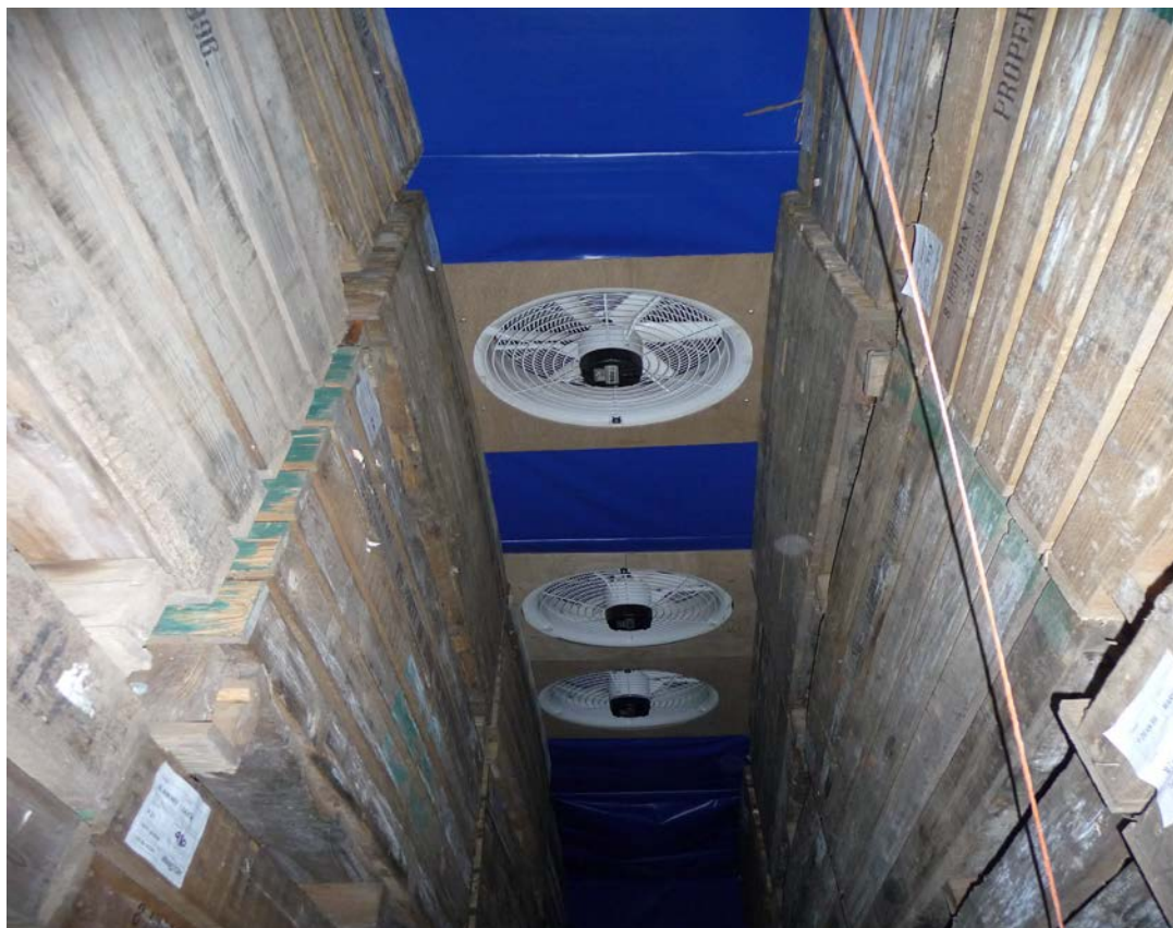
Figure 1. Recirculation fans mounted on a plenum drawing air from the store headspace into the plenum in positive pressure plenum treatment.
