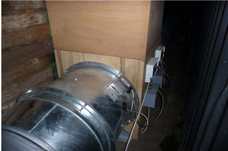
Figure 2. Fans being used to extract fog from a plenum in negative pressure plenum pattern of application.
