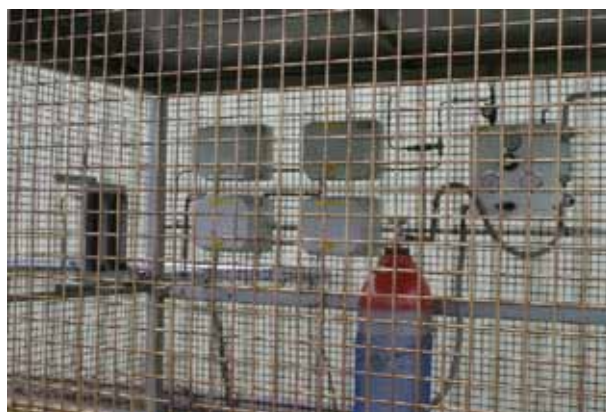
FIG. 2. ‘CAGED’ ETHYLENE CYLINDER STORAGE FOR BIOFRESH CONTROL SYSTEM.
