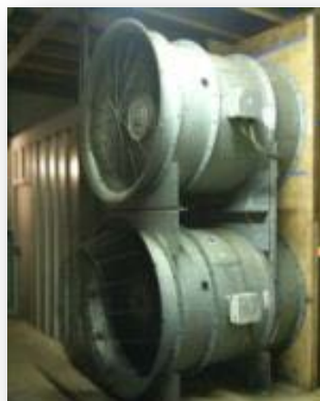
Figure 6.5.6 - Main store fans
