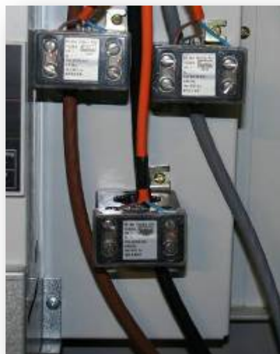
Figure 6.1.2 - Current transformers (CTs)
