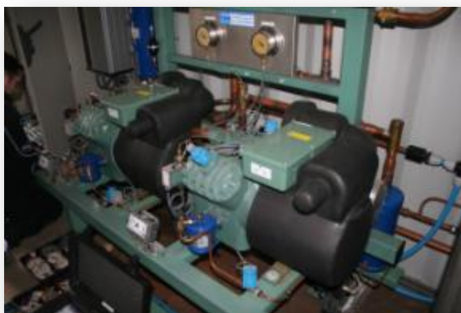
Figure 6.5.2 - State of the art refrigeration plant
