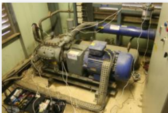
Figure 6.5.3 - Store 5 refrigeration plant
