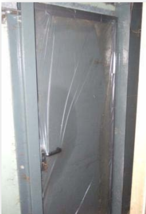
Figure 3.5.7 - Personnel door sealed from inside
