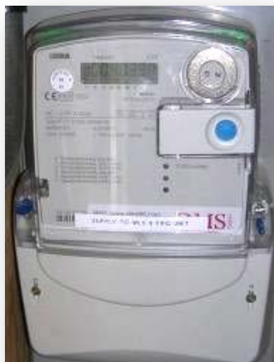
Figure 6.1.1 - Electricity meter as installed
