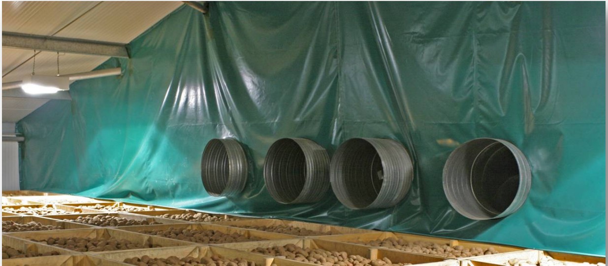
Figure 3.9.1 - Air divider curtain fitted in store
