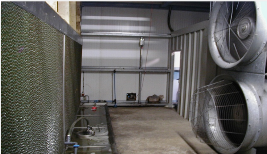
Figure 3.10.1 - Example commercial humidification system in test Store 7
