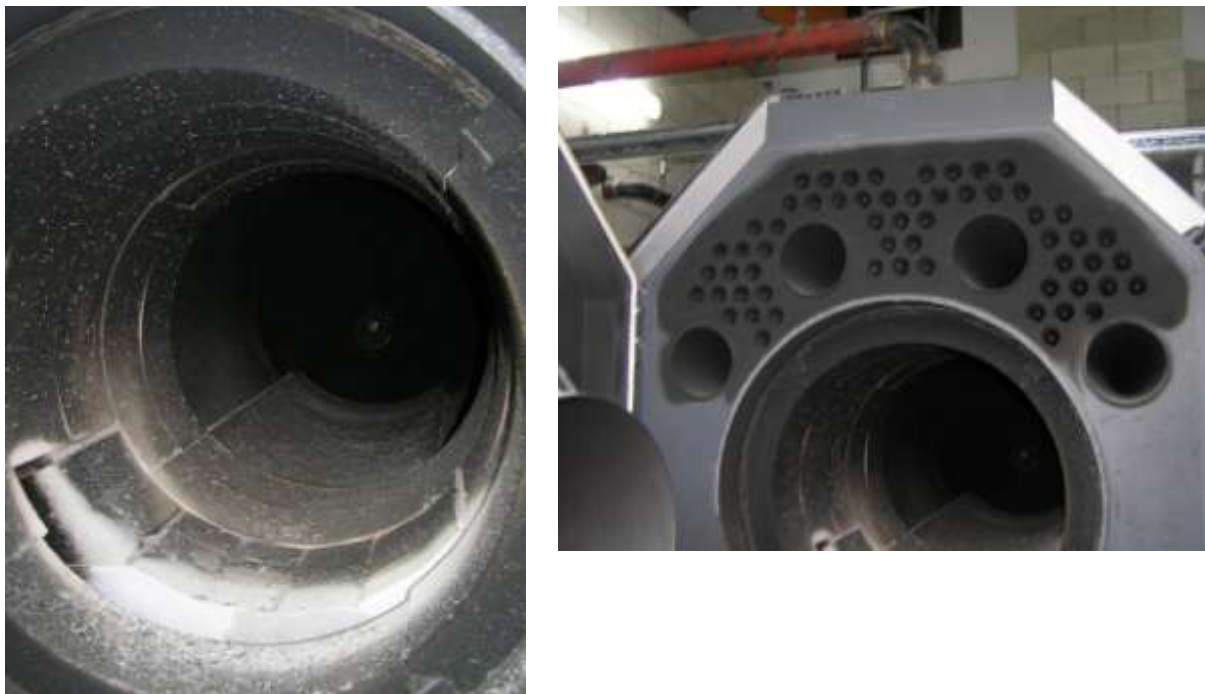
Figure 9. Combustion chamber in a Kob boiler
