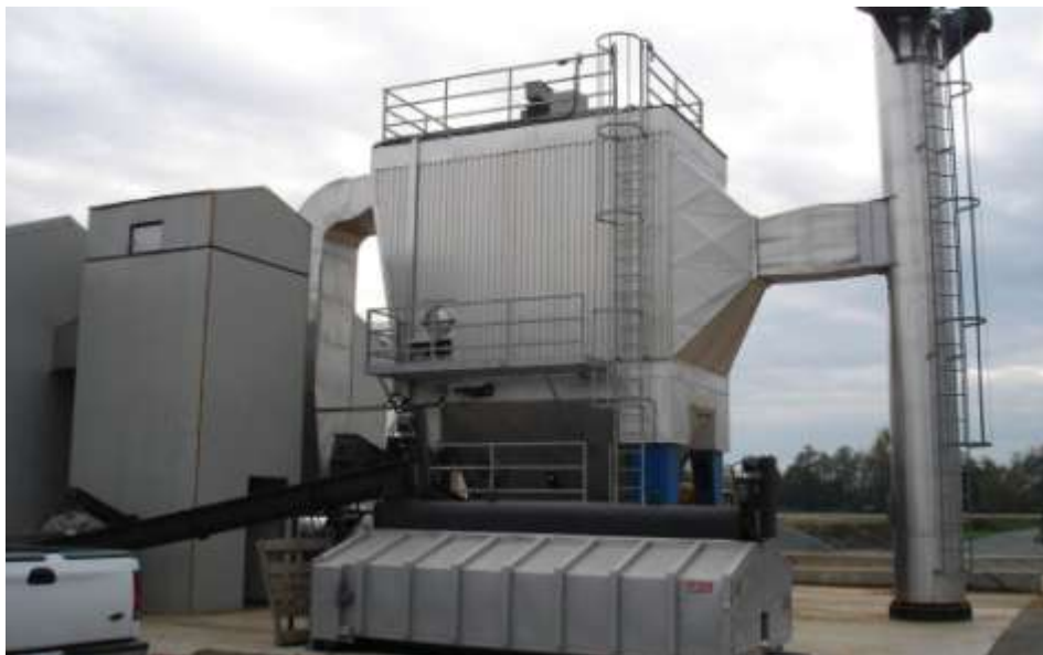
Figure 13. Dry ESP on a 5MW boiler
