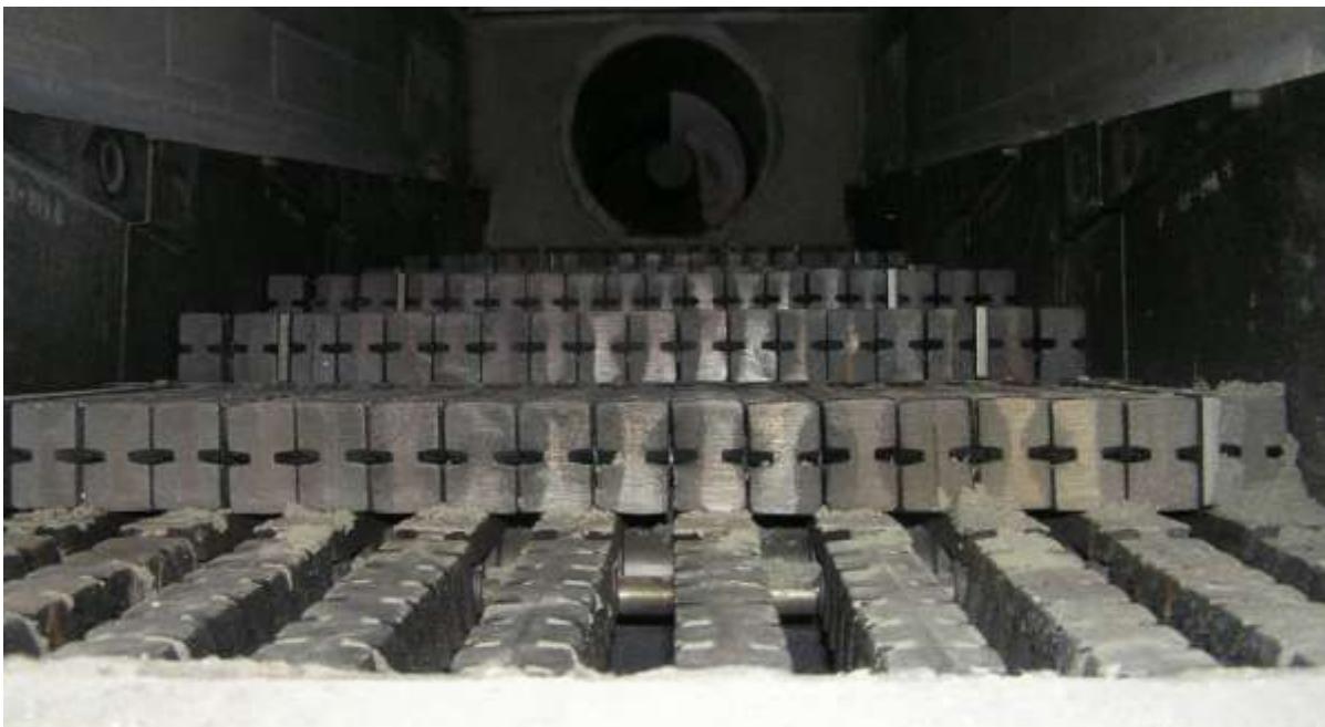
Figure 7. A moving stepped grate
