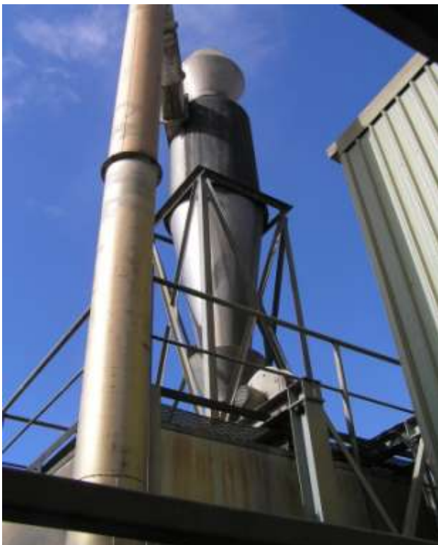
Figure 10. Cyclone on a fuel supply
