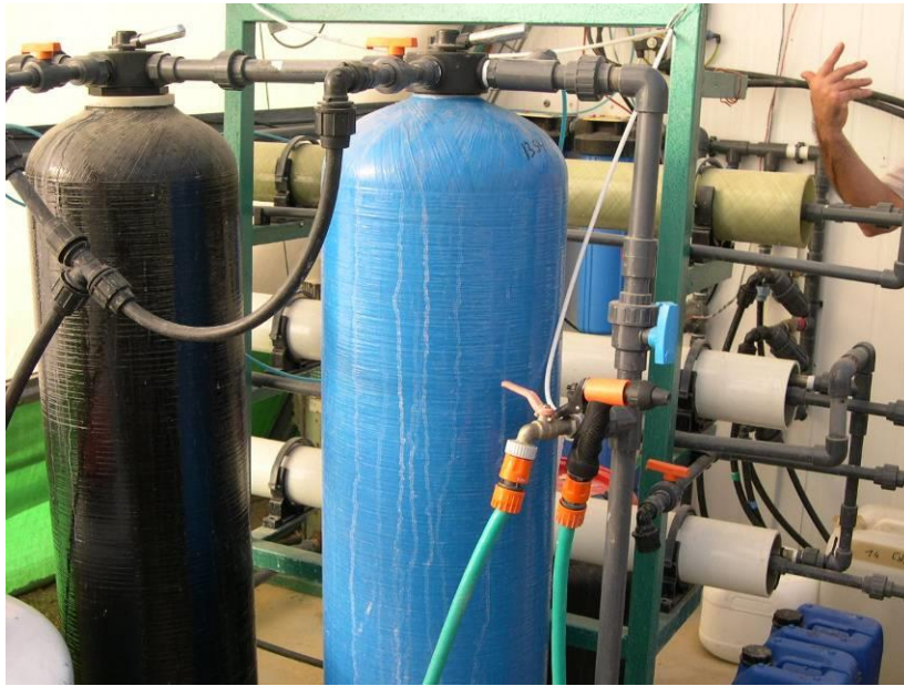
Plate 9: View of the reverse osmosis units used to remove all contaminants, including base nutrients and pathogens, from the water supply.
