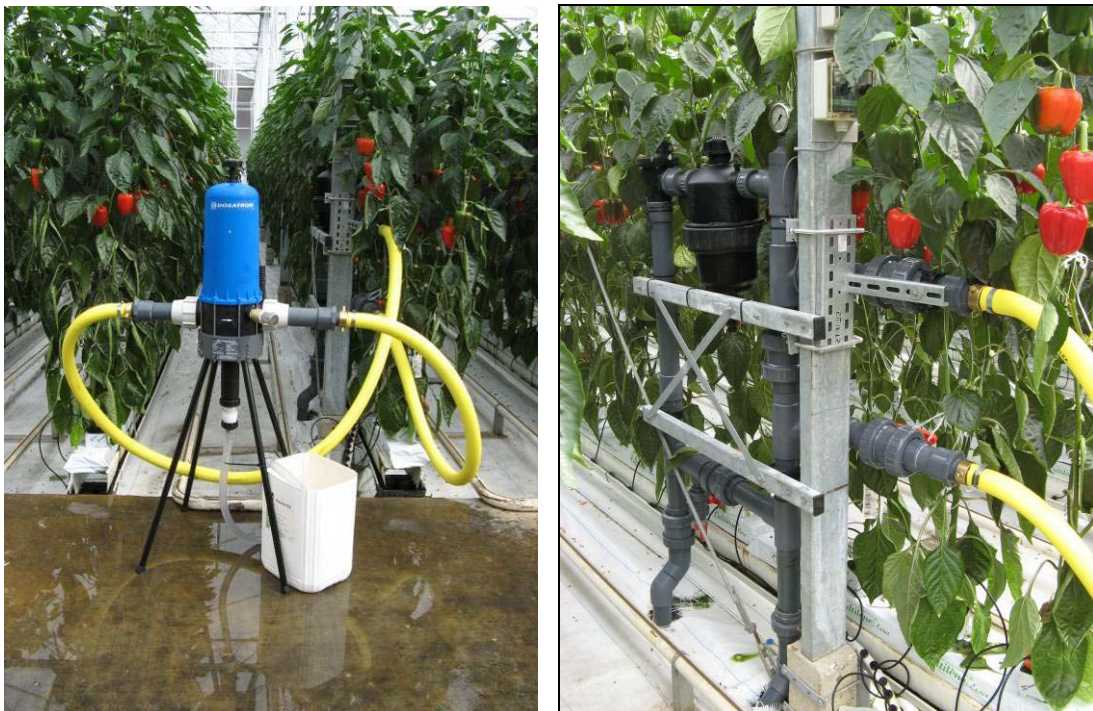
Figure 15. Dosatron in situ showing stock tank (white container) and connections to manifold
