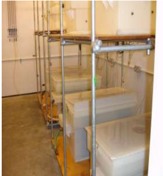
Storage cabinets – refrigerated store
