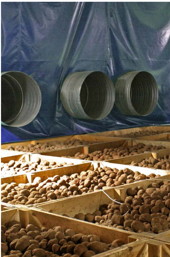
Figure 3. An air separator curtain boosts ventilation efficiency significantly by preventing short circuiting
