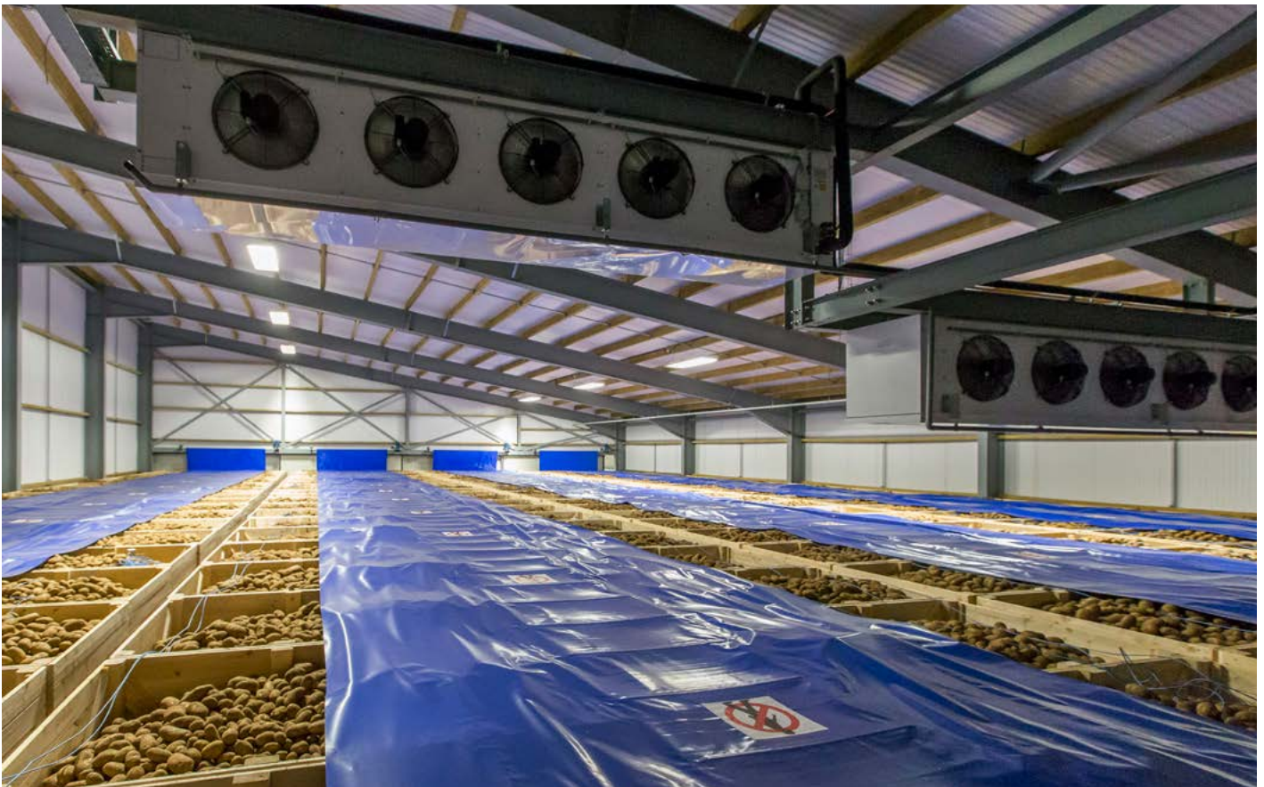
Figure 4. Lateral suction is a positive ventilation option for box storage
