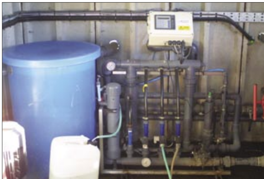
5 A typical acid dosing system
