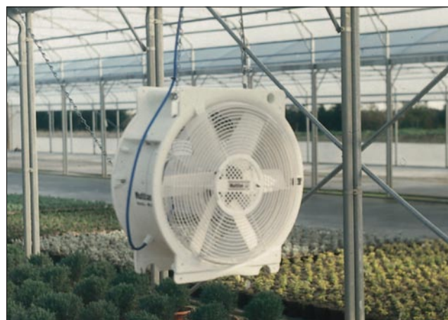
12 Fan ventilation is an effective way of providing good air movement to help combat Botrytis , particularly in larger structures
