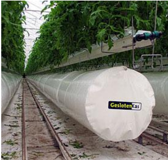
Fig 3 – The air distribution system used in the Dutch sealed greenhouse project.
