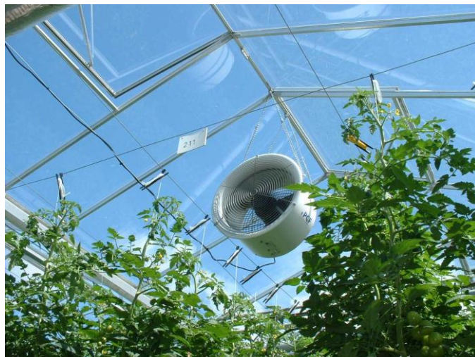
Figure 2 – An example of a horizontal air circulation fan
