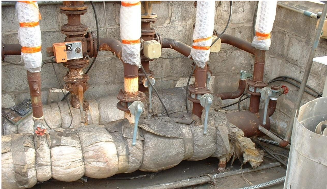
Poor insulation costs energy
