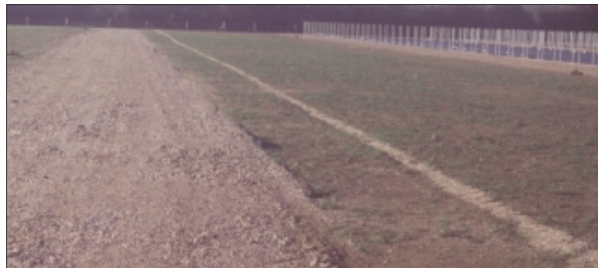
9 Prepare land thoroughly when installing capillary watering systems including accurate levelling of your site
